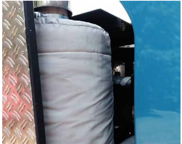
Insulation of a particulate filter
